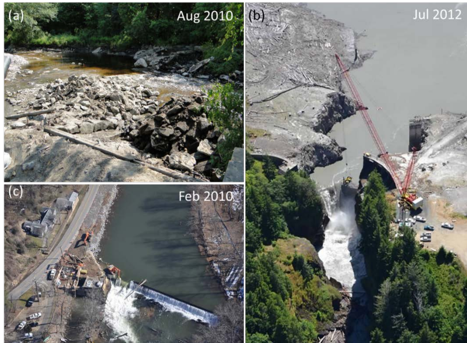
Figure 5. (a) Lower Shannock Falls Dam Removal and Fish Passage project was conducted as part of a wider strategy to restore natural conditions at the Pawcatuck Watershed Start (photo by Chris J. Fox, Wood Pawcatuck Watershed Association, Rhode Island). (b) Elwha river dam in the state of Washington after removal and (c) Dillsboro Dam on the Tuckaseegee River in North Carolina being removed (photos by Andy Coburn, Western Carolina University).
