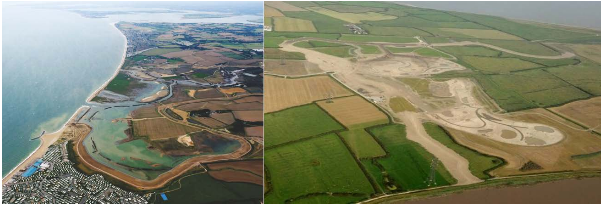
Figure 26. Managed realignment at Medmerry (left), West Sussex, southern England, was breached in November 2013; it will create around 320 ha of intertidal habitat once completed. The Steart Coastal Management Project under construction (right), Somerset, southwest England, is the largest managed realignment site in the UK to date (over 400 ha); breach is to occur in 2014.
