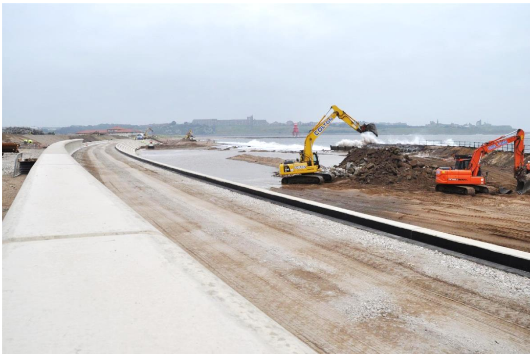
Figure 12. Realignment of the seawall at Littlehaven Beach in 2013 was an integral part of the local regeneration plan to increase the aesthetic and amenity value of the beach frontage, in addition to improvement of coastal protection (Photo from Steve Burdett, courtesy of Royal HaskoningDHV).
