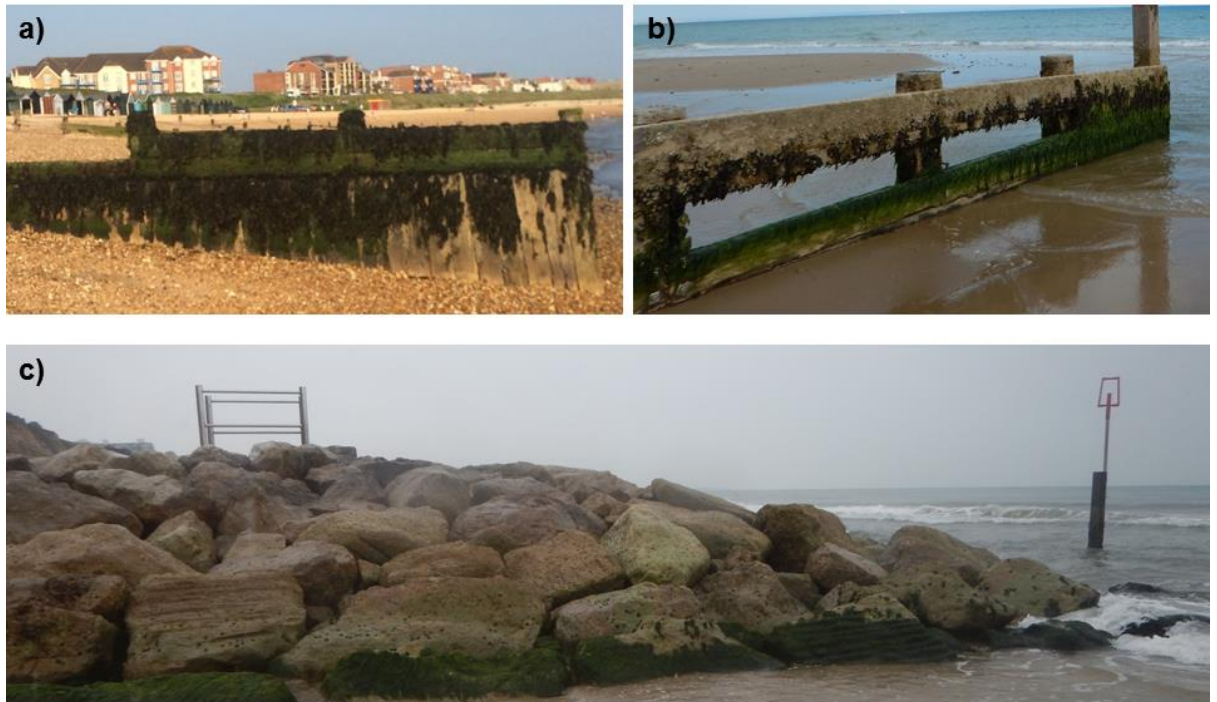
Figure 2.1 Groynes sampled along the south coast of England a) wooden groyne with fucoid canopy cover in Region 2, b) damaged wooden groyne with planks missing in Region 1, c) rock groyne toe in Region 1.
