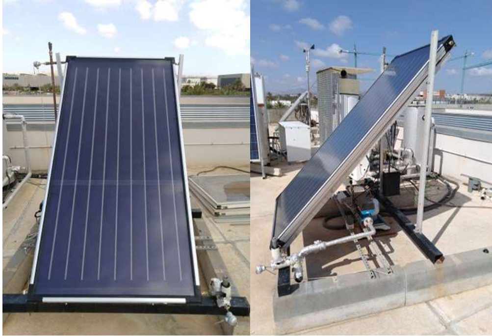
Fig.2. Solar testing facility.
