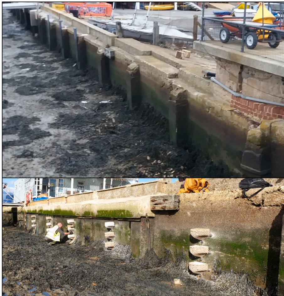
Fig. 2. Top: the seawall in 2017 prior to rockpool installation. Bottom: the seawall during rockpool installation in October 2020.
