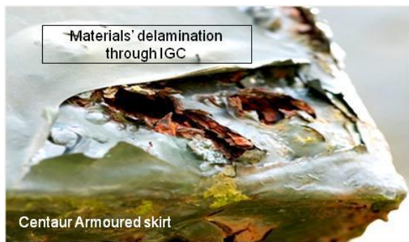
(c) Inter-granular corrosion in the armoured skirt
