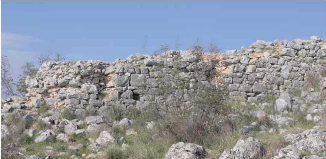
Fig. 25. Early Byzantine curtain wall on Kourtikiano hill (between Tower 4 and Tower 5 ), as seen from outside (looking towards west). Photograph by I. Randall.
